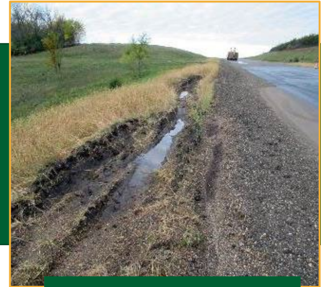
Erosion Control Problems
