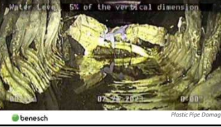
Plastic Pipe Damage
