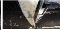
Severe cross frame distortion
