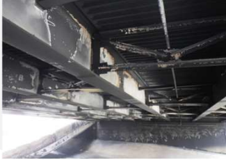
Underside of the southbound structure, looking back. Note the heavy soot staining
